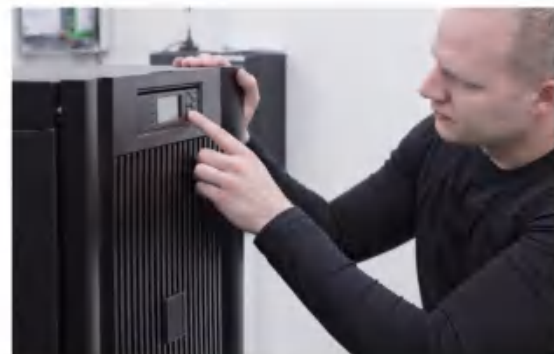
UPS power supply systems
